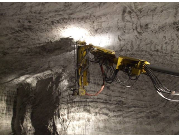
After scraping, 1.2 m long bolts are inserted into the ceiling for stability.
