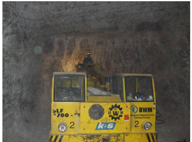
The rock face being drilled and charged with explosives for blasting. The blasting is carefully controlled to ensure the correct detonation pattern occurs to allow thorough loosening of the rock material.
