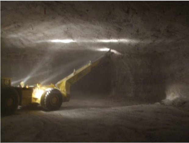
After the freshly blasted ore is removed, the ceiling of the mine is scraped to remove any loose rock debris. This process ensures that no loose rocks will fall causing danger at a later stage.
